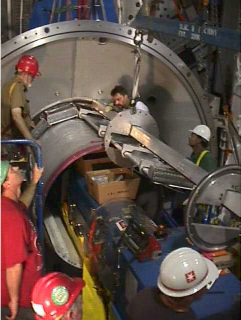
Figure 15: Installation of a barbox into the BaBar detector. Not seen in the figure is the cantilevered support arm which supports the installation fixture above the accelerator components.
