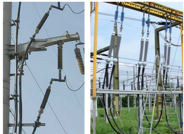
Fig. 7: 123 kV dry slip-on terminations installed on a mast or used for temporary link.
